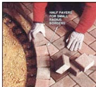
12. USE HALF PAVER for bordering tight circles. Smaller pavers cut down on the size of the pre-shaped gaps between each piece.
