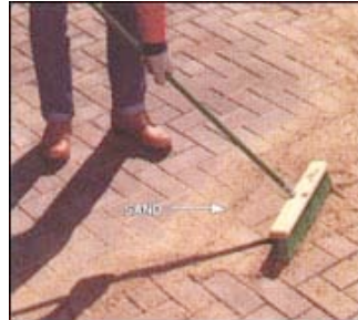
15. SWEEP COARSE, DRY SAND between cracks of pavers to lock together and fill voids. Repeat with more dry sand in a few days.
