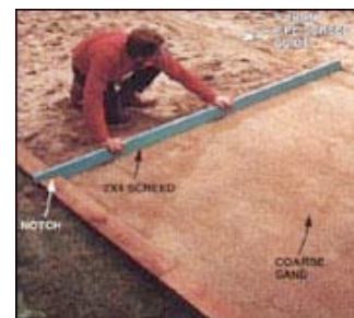
8. SPREAD AND LEVEL a 1 inch bed of sand over compacted subbase. Pipes provide a guide for dragging the 2x4 screed board across.
