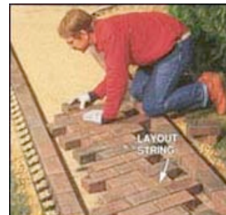
LAY THE PAVERS using a string guideline. Cut and install pieces that build up to the border later.
