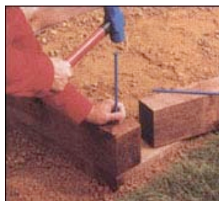
7. INSTALL LANDSCAPE TIMBERS for edging in areas where you need to change levels or step down. Be certain to overlap corners.
