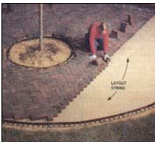
10. CONTINUE LAYING PAVERS using a layout string to keep them in line as you work. Put a gap between pavers or tap them tighter to stay in line.
