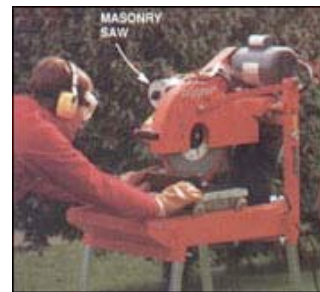
13. CUT PAVERS on masonry saw. Saw has a built-in sliding carriage for moving pavers past the blade. Recirculating water keeps blade cool and lubricated.
