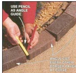
INSTALL THE BORDER marking and cutting other paver at an angle at curved areas.
