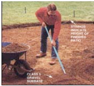
4. SPREAD CLASS 5 subbase to a depth of 4 inches over entire patio area and 8 inches beyond. Measure down from guide strings to establish uniform height of subbase.
